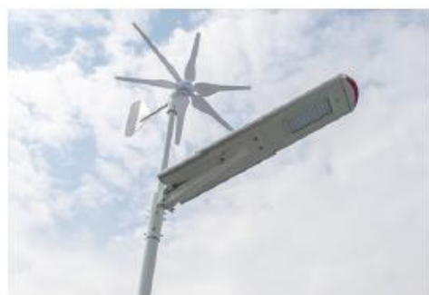
12. Check all the screws fasten, and make the light pole upright, installation finish
