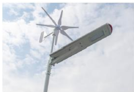
12. Check all the screws fasten, and make the light pole upright, installation finish
