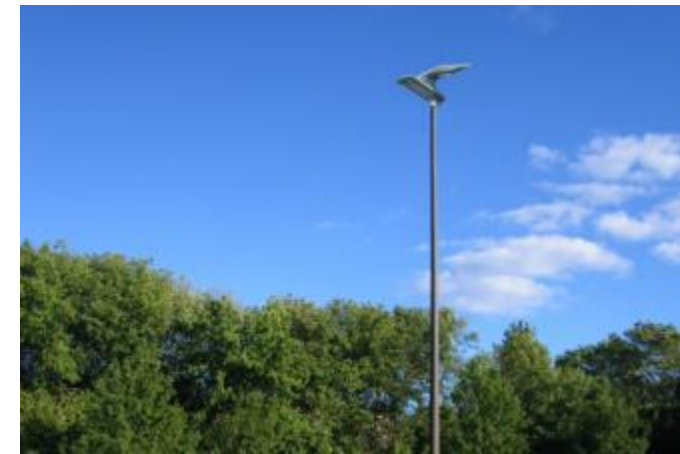
Open Parking Lot Lighting
