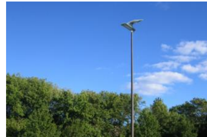
Open Parking Lot Lighting
