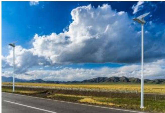
Traffic Road Lighting
