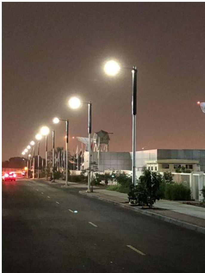
Solar LED Streetlights in Dubai, UAE
