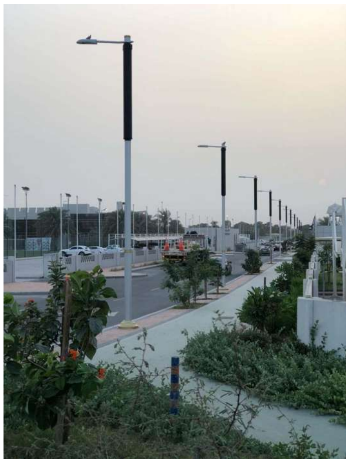
Solar LED Streetlights in Dubai, UAE
