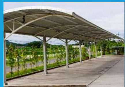
Solar Parking Canopies
